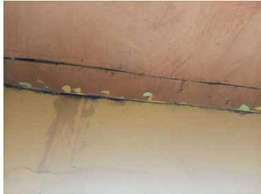
Water damage and leakage
