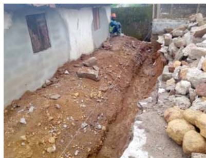
The woman's home with repairs. The areas of new concrete are where the house caved in.
